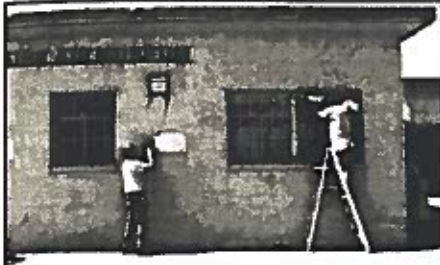
President Jim Chichetto and Les Shaw prepare the building exterior for painting.
